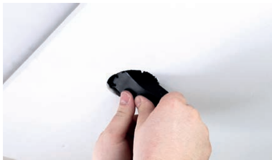
2 - quick connection box is placed over the 68 mm cut-out in the cavity
