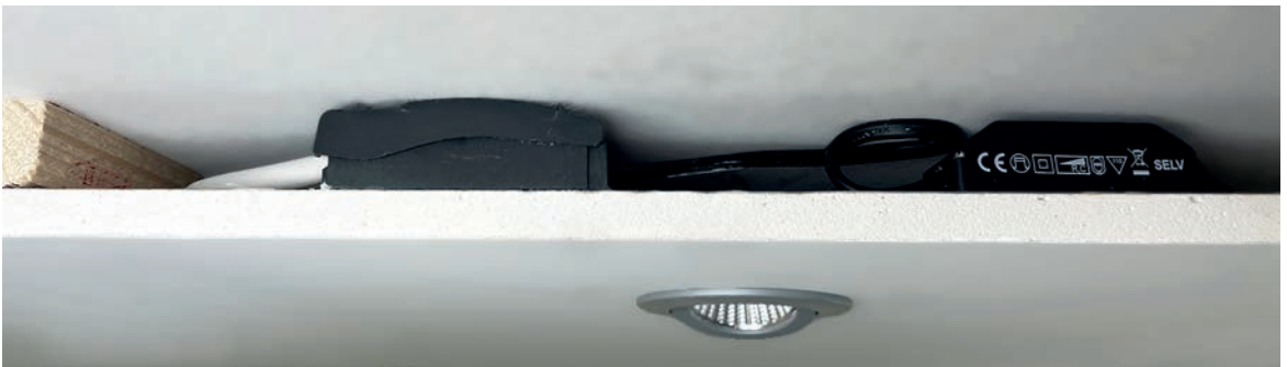
6 - The result: a compact installation with a swivelling spot, a dimmable power supply unit and the option of through-wiring in the ceiling cavity - ideal in refurbishment areas.
